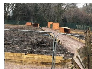
Sheds at the new site at Aldershot Road blown over by Storm Eunice
